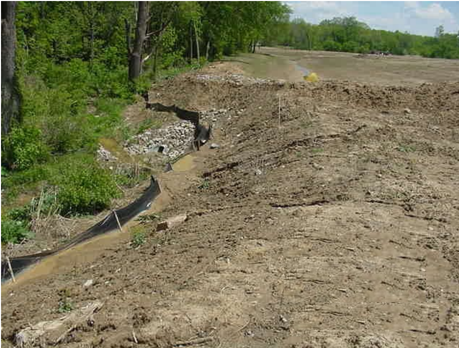
Silt fence in need of repair
