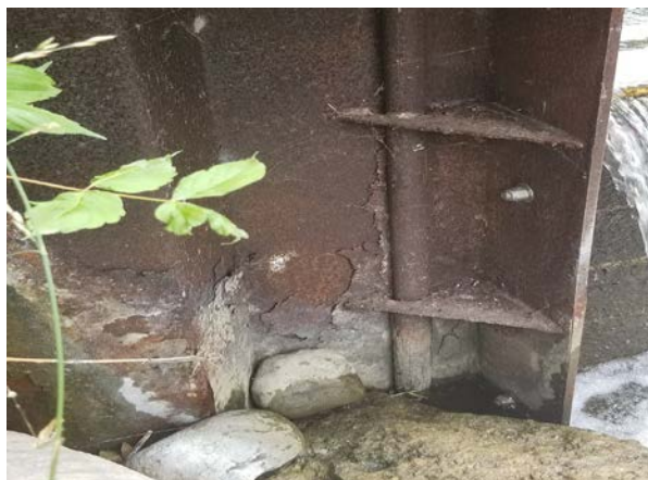
Oxidation of metal gate components (West side)
