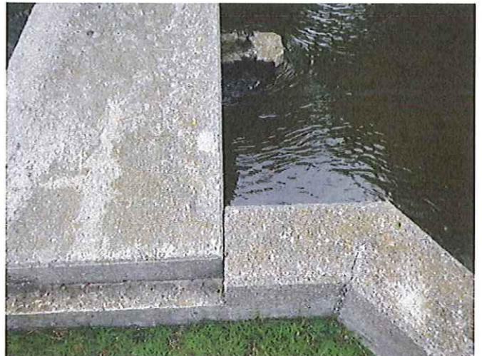
Crack-Southeast Side; Shows walkway shifted slightly
