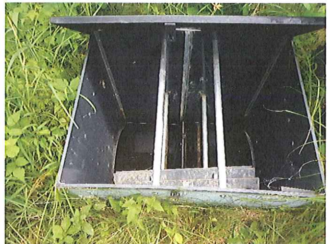
Inside Control Structure
